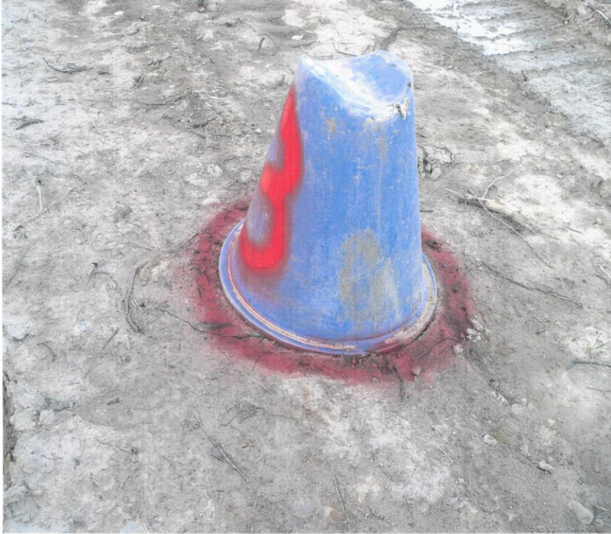
Figure 2. A pipe support cone.
