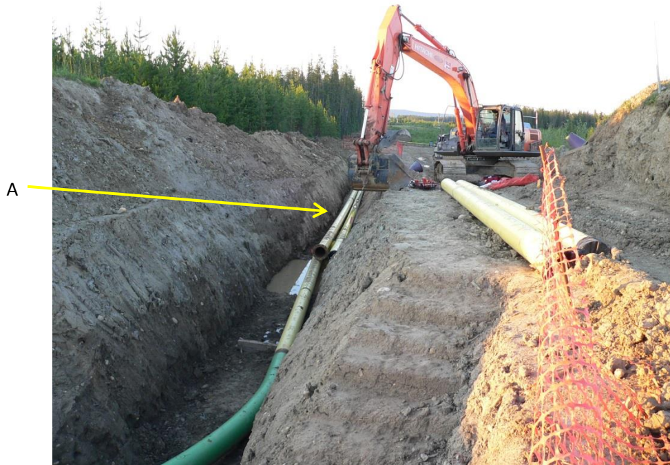
Figure 1. The image shows the trench where the Foreman was struck. Also shown are the pipes, excavator, and the blue pipe support stands.
