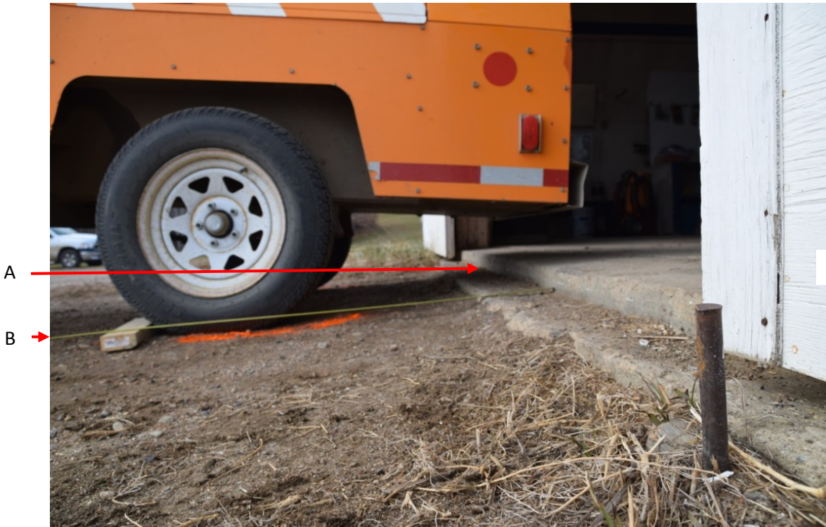
Figure 3: The transition area between the concrete floor of the workshop and the gravel approach.
